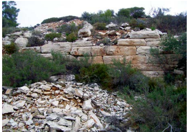
Fig. 17: The ashlar multifunctional wall at the SW slope of Vouno Michali (photo by A. Kapetanios).
